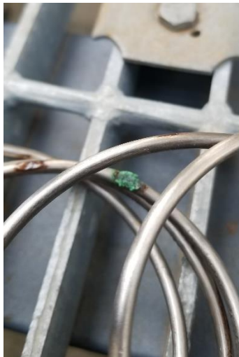
Exhibit 27. Corrosion on temperature probe.
