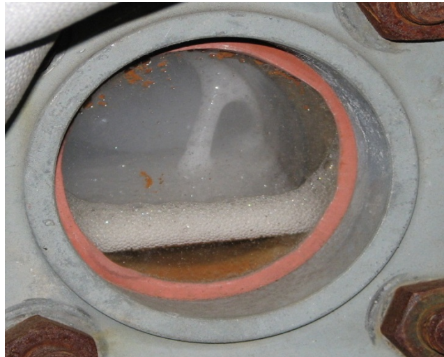
Figure 6. Foaming Observed through Wash Tower Port
