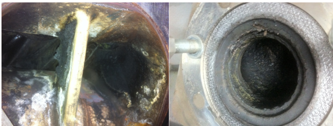
Figure 7. Pictures of the feed compressor components showing particulate buildup and corrosion.
